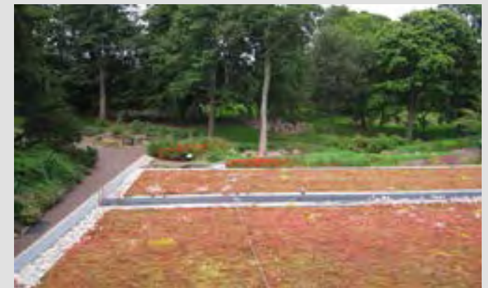
Extensively green roof—Botanic Gardens The planting on this green roof helps integrate the building into its surroundings
