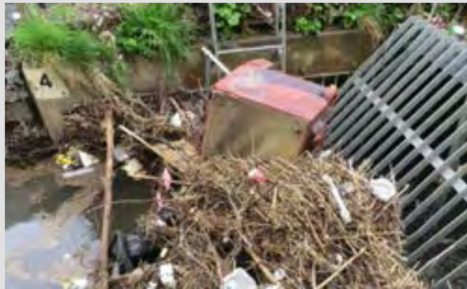
locked up culvert
